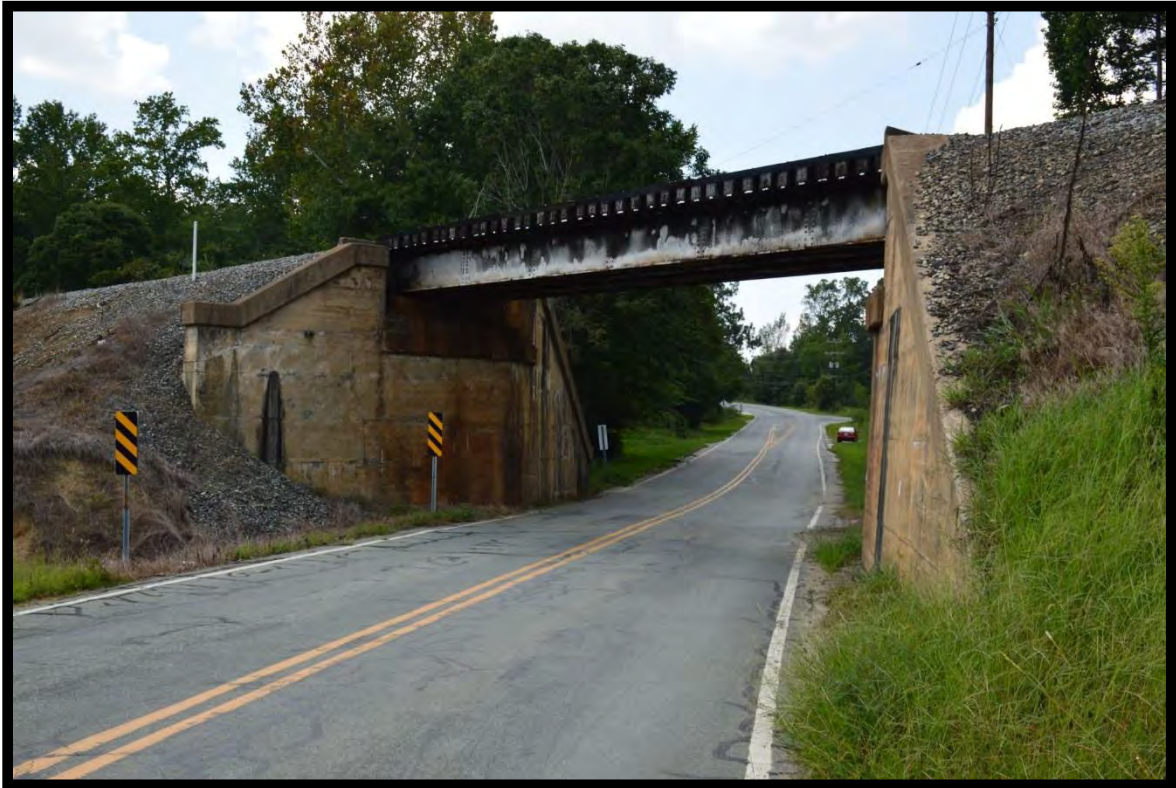
Figure 17: Overpass Carrying the North Carolina Railroad (GF8976) over Old Burlington Road, Looking West.
